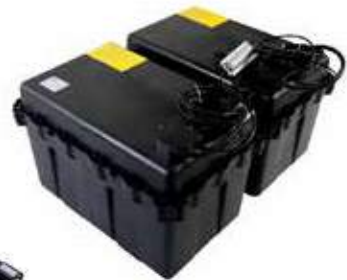
Battery on Ground in IP68 Box
